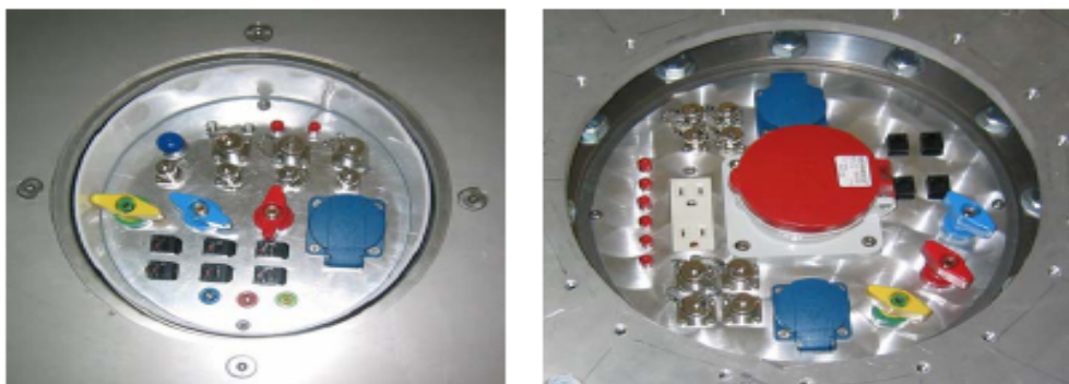
Figure: Power supply in the centre for EUT
